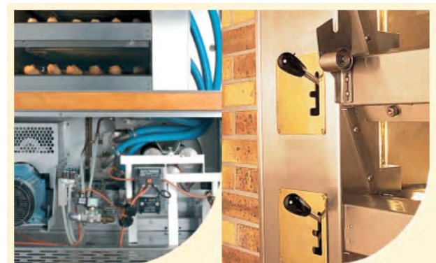
Steam generator located near to the burner.
