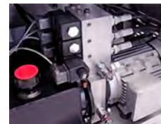
Big tank and double sealing between tank and hydraulic unit
